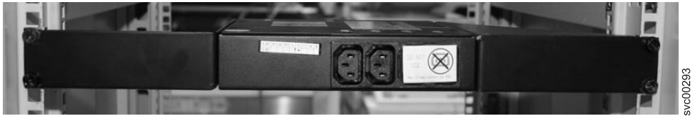
Figure 25. Positioned in rack
