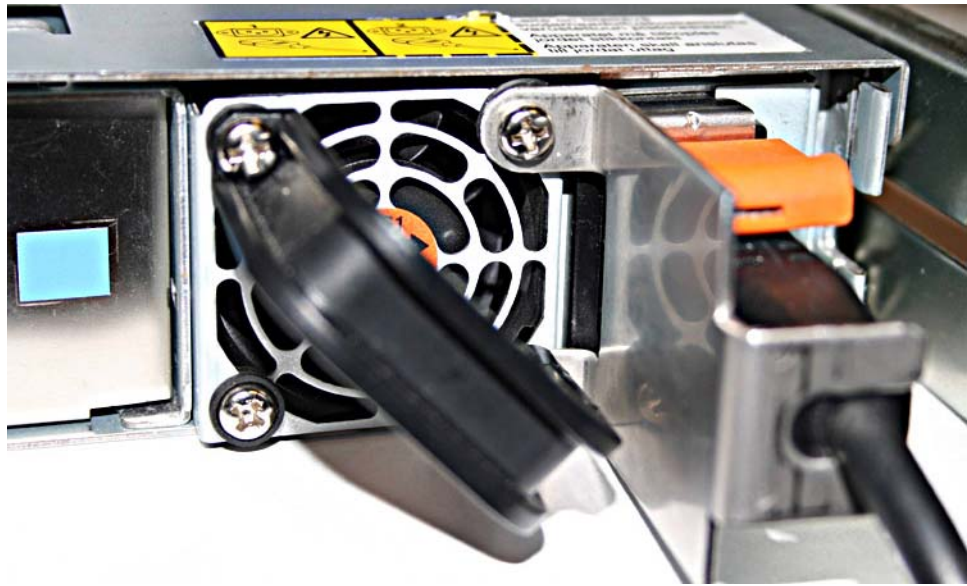
Figure 66. The SAN Volume Controller 2145-8G4 with cable retention bracket option A attached
