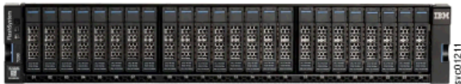
Figure 1. Front view of the control enclosure
