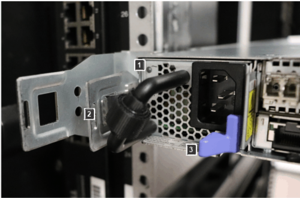
Figure 70. Features of a power supply unit
